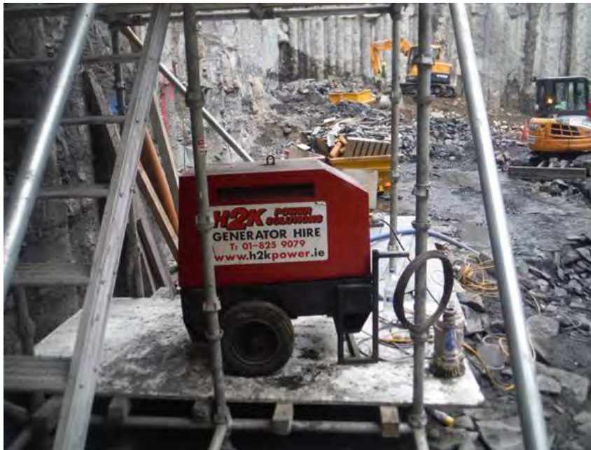
Check Location and Exhaust Fumes
