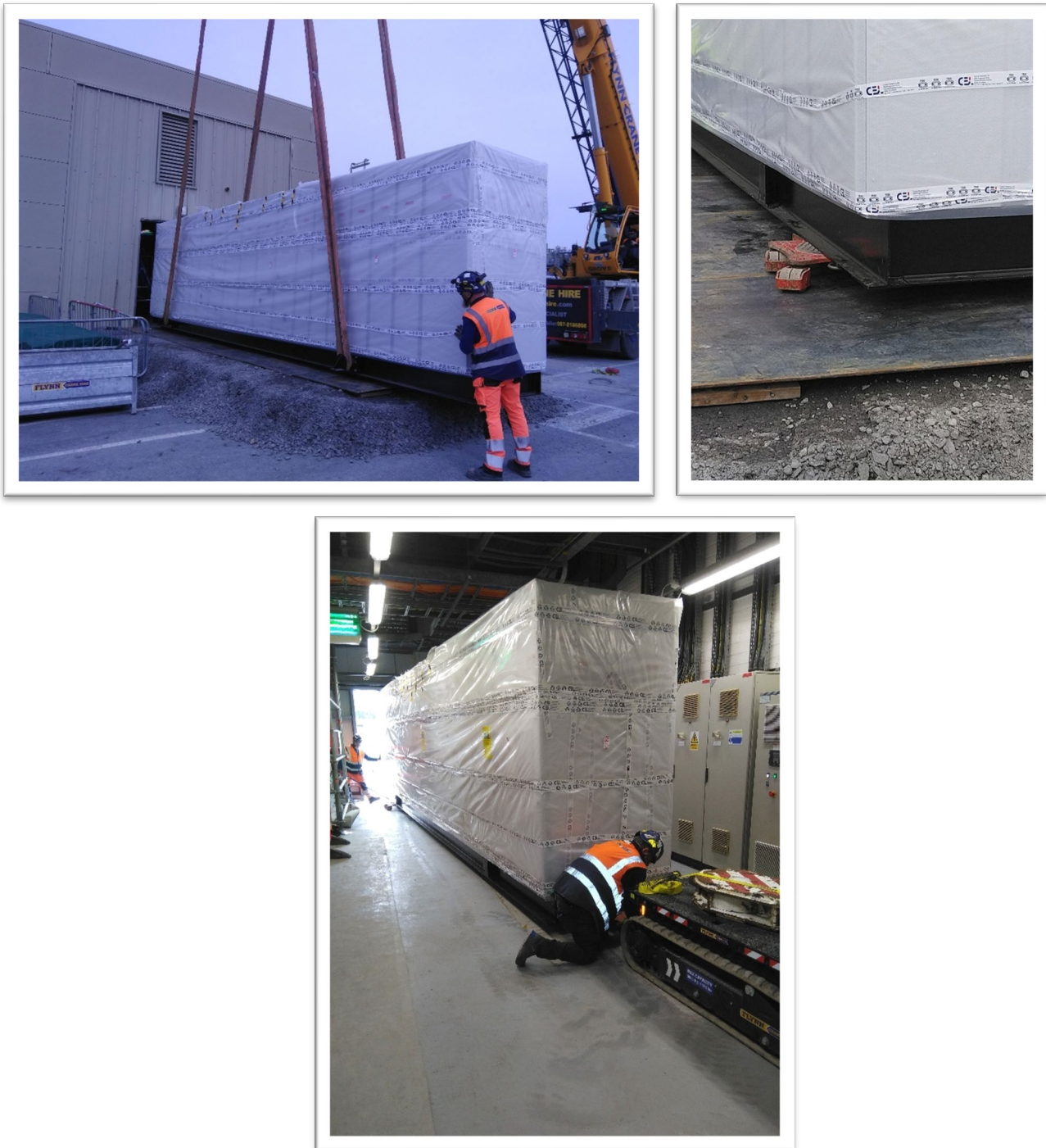
Figure 17 - Examples of Brownfield Installation
